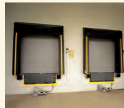
Rolling Service Doors
